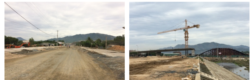
Phong Chau Road fronting Parcel 2 & new bridge over Quan Truong River, 30 June 2016
